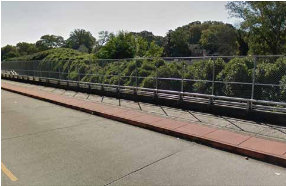
A modified bridge on Westview Dr SW in Atlanta to accommodate a 10' wide multi-use trail
